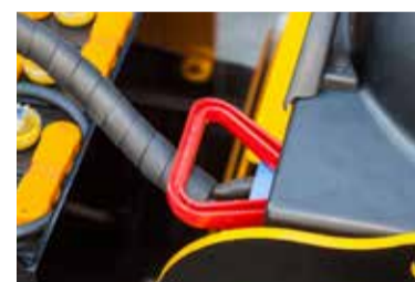
Battery disconnect lever
